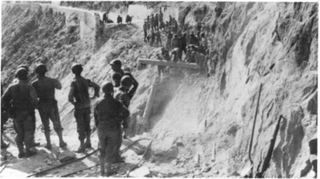
The 10th Engineers begin to “hang a bridge in the sky,” 13 August 1943.
