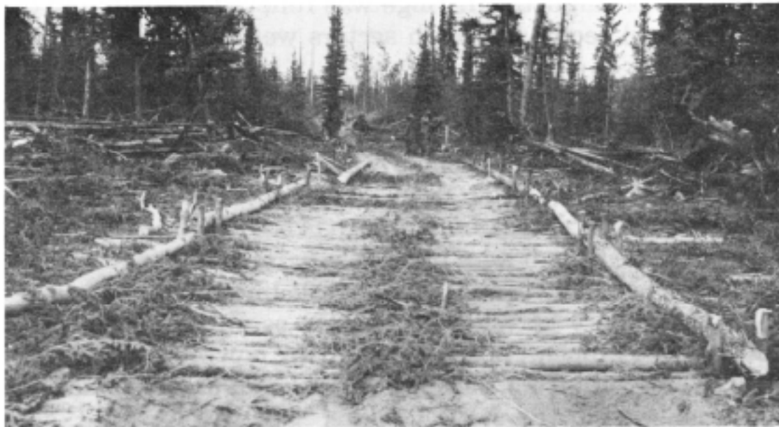
Corduroy roads, such as this one built by the 93d Engineers near Little Atlin Lake Yukon Territory, were necessary in boggy areas and to cover permafrost sections to prevent thawing.
