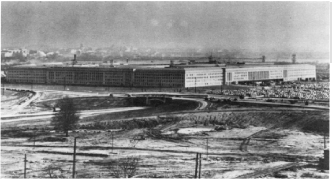
Pentagon construction, northeast exposure shows part of the south parking and access roads, 30 November 1942.
