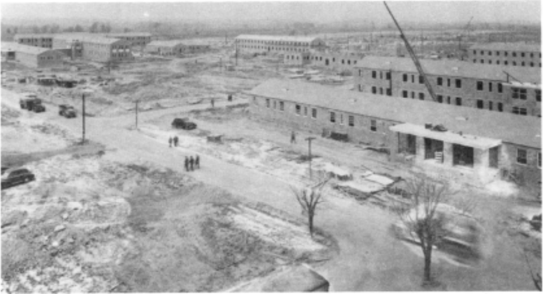
Semipermanent hospital buildings in various stages of completion, Camp Atterbury, Indiana, 25 April 1942.
