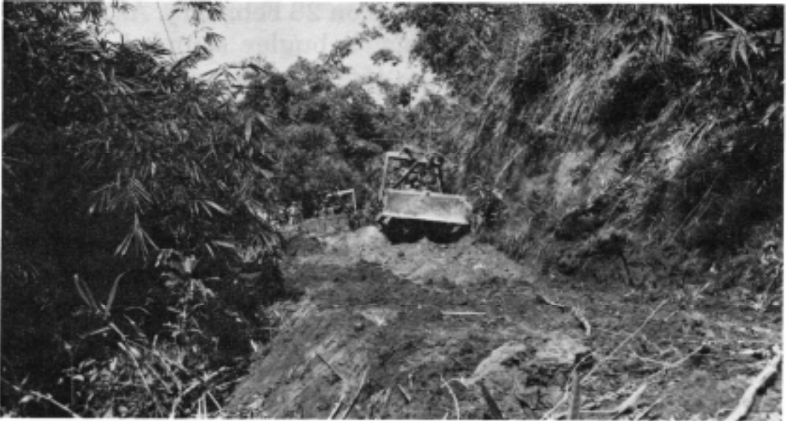
Bulldozers clear a slide in Burma, as engineers construct the Ledo Road.
