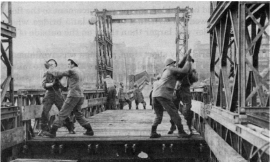
Engineers lift the bascule span of a class 70 Bailey bridge. (Engineer School Library)
