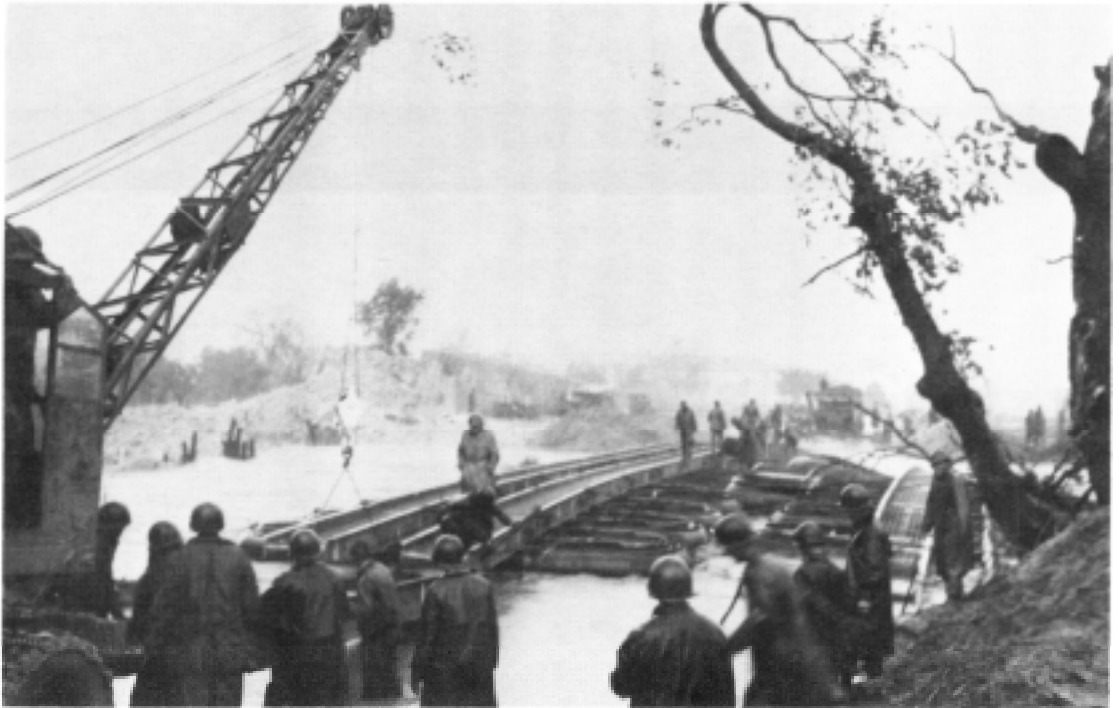
The 16th Engineer Battalion adds steel sections to protect a ponton bridge against the rising waters of the northern Volturno River
