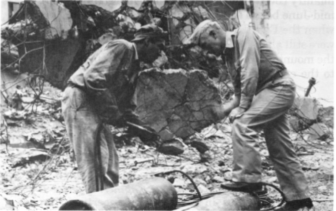
Engineers cut steel reinforcers in concrete from the Manila City Hall building. Here Major General Hugh J. Casey speaks to PFC Perry Alexandeer, a welder with the 1879th Engineer Aviation Battalion, 23 March 1945.
