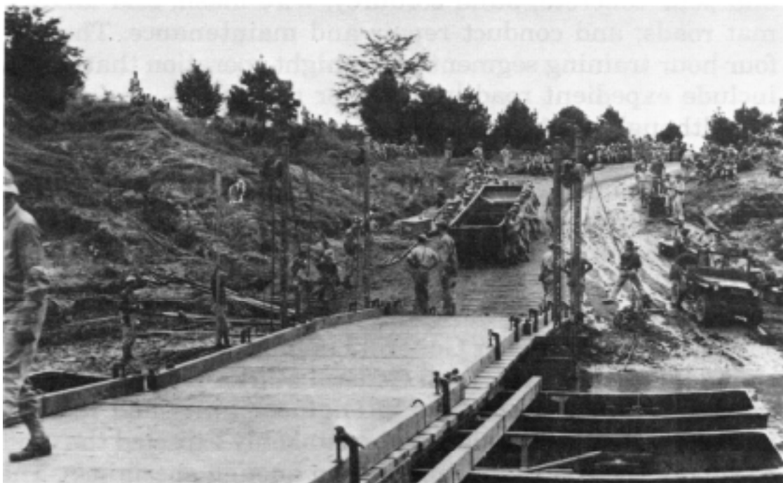
Engineers build an assault boat ponton bridge (10-ton capacity) with two fixed steel trestles on the shore
