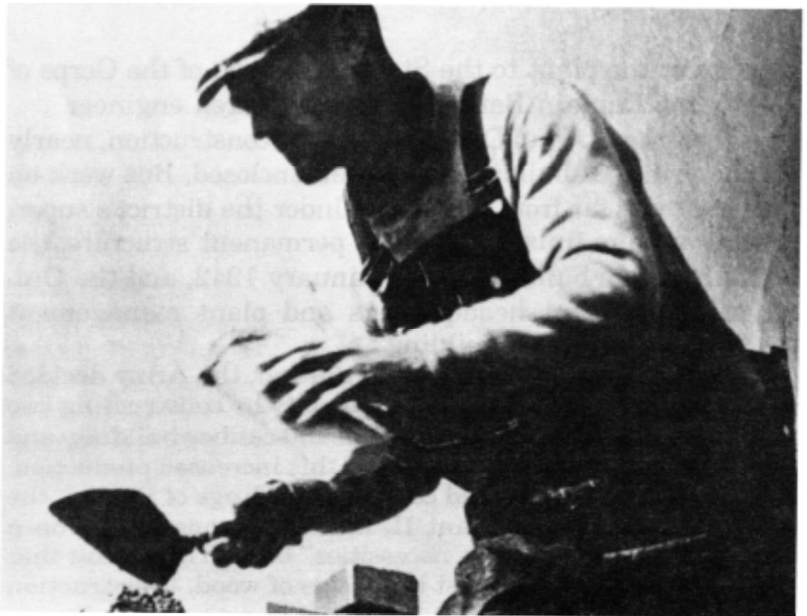
Brick laying at the Twin Cities Ordnance Plant. (St. Paul Pioneer Press, 26 October 1941)
