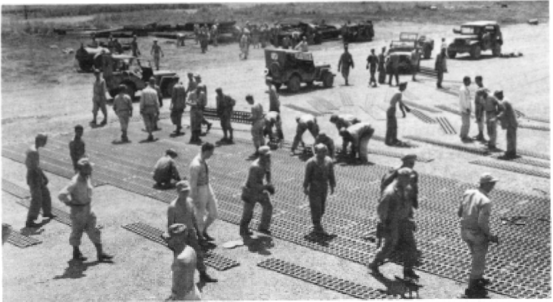
After rolling and compacting an airstrip in the Markham Valley, New Guinea, aviation engineers place pierced steel plank on the 7,000-foot runway.
