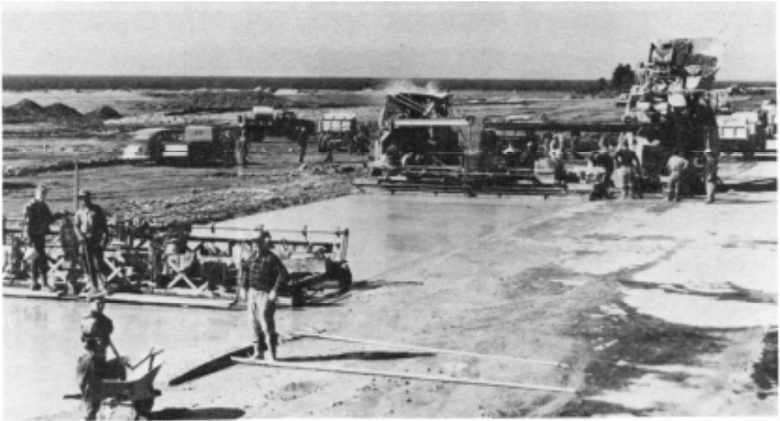
Pavers work both ends of a 25-foot-wide slab on Runway 2 at Harmon Field on Newfoundland's west coast.
