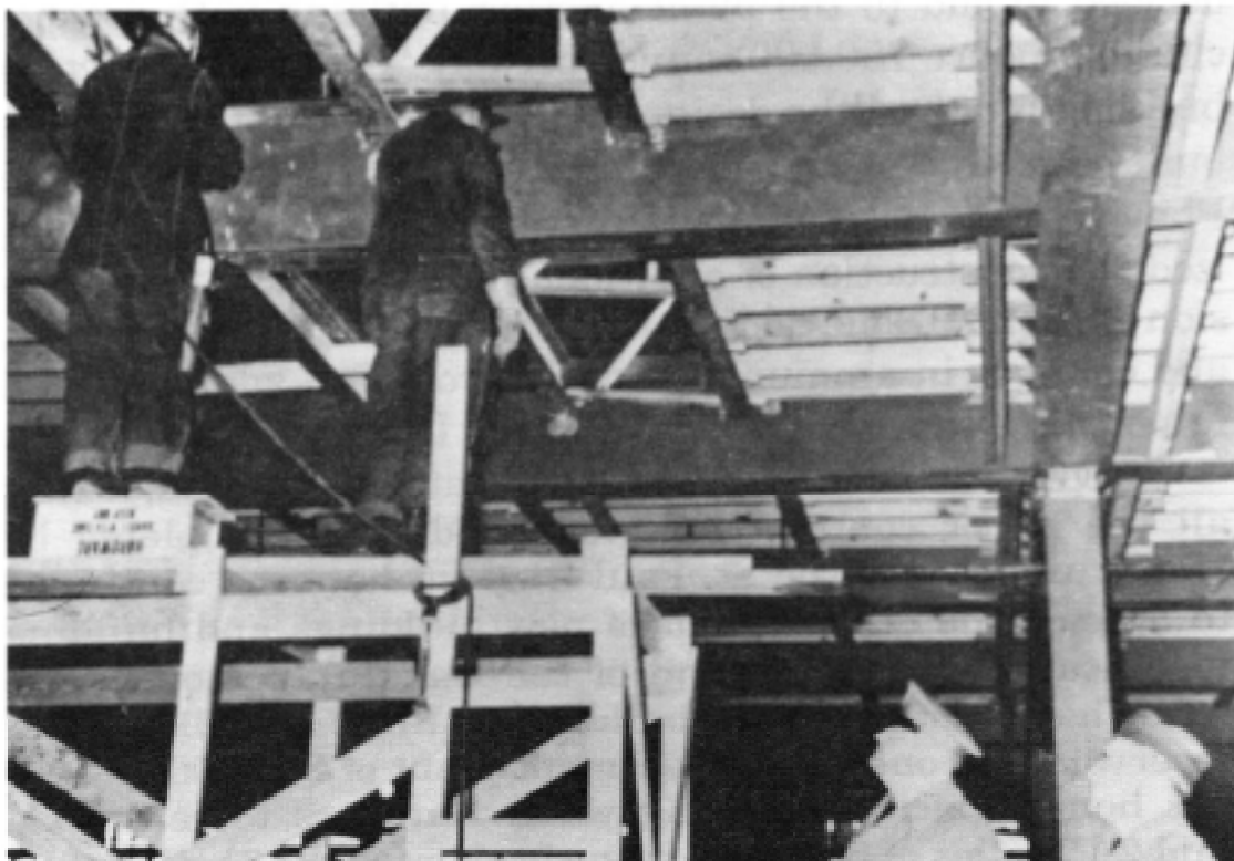
Major Lynn C. Barnes (far right) inspects work at the Twin Cities Ordnance Plant.
