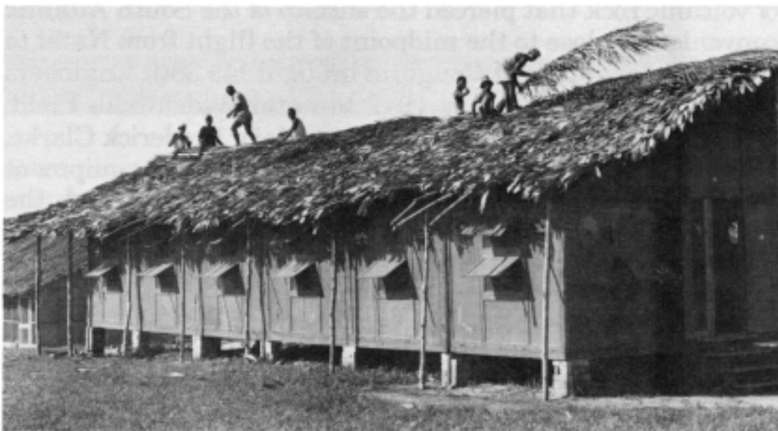
Local workers complete the thatched roof of enlisted men's barracks at Roberts Field, Liberia, May 1943. (U.S. Air Force, National Air and Space Museum, Smithsonian)
