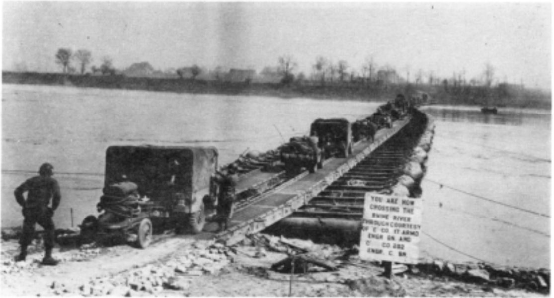
Overnight the engineers built this ponton bridge spanning the Rhine River in the vicinity of Wallach, Germany, 25 March 1945.
